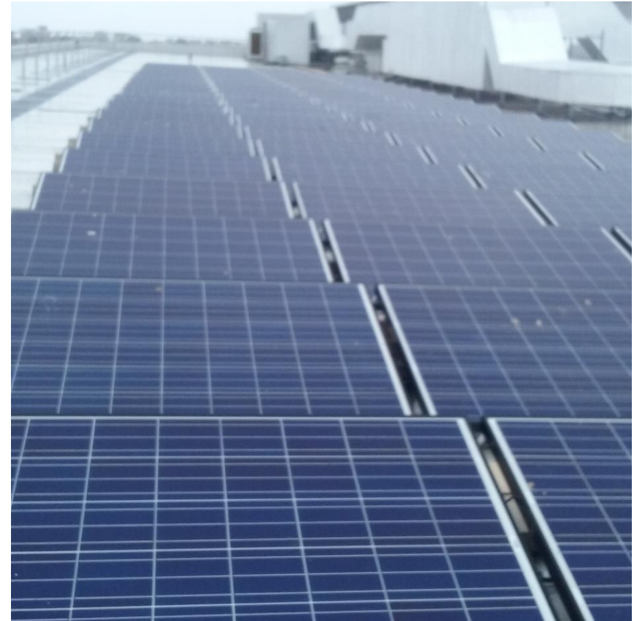
Figure 0.0.1: Rooftop solar panels
